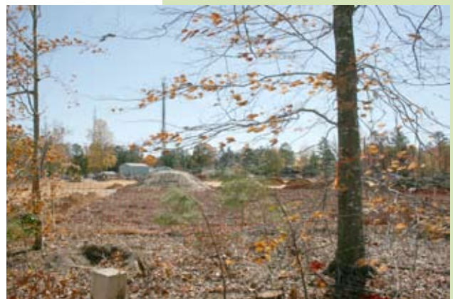
Another view of the construction site seen through a portion of the Monticello buffer.
